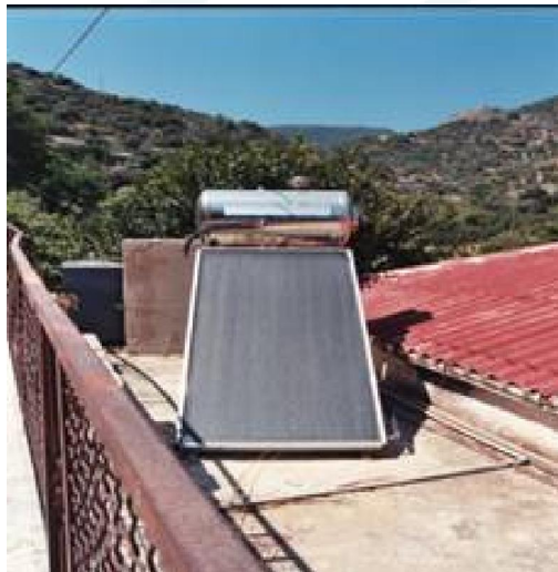
Solar thermal collector, Greece
